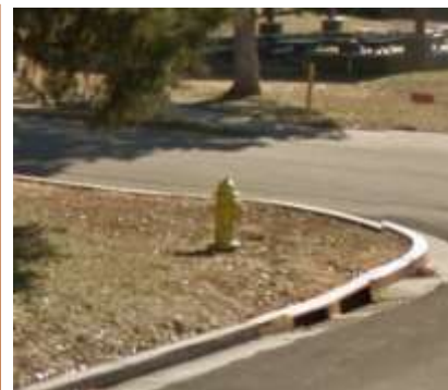
Fire hydrants provide needed water to fight fires and allow water lines to be flushed to keep the water clean. They can also be tested to check the water pressure and flow in the area.
