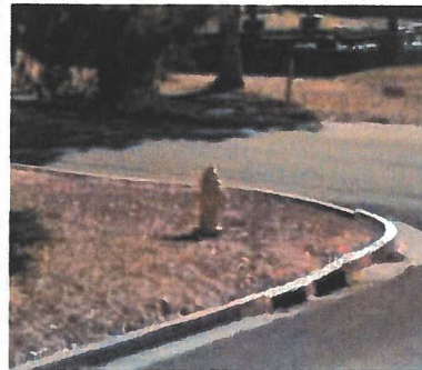
Fire hydrants provide needed water to fight fires and allow water lines to be flushed to keep the water clean. They can also be tested to check the water pressure and water flow in the area.
